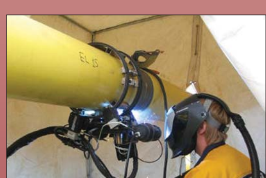
27cm (10") Gas Pipeline - Estonia
