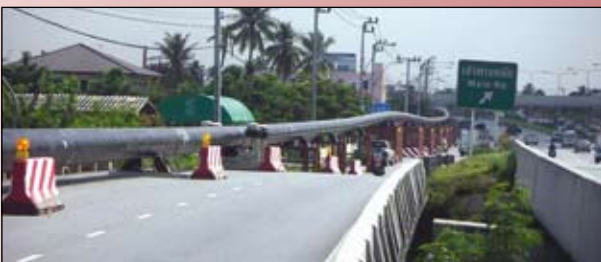
76cm (30") Gas Pipeline - Bangkok, Thailand
