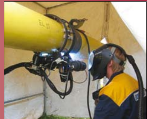
27cm (10") Gas Pipeline - Estonia
