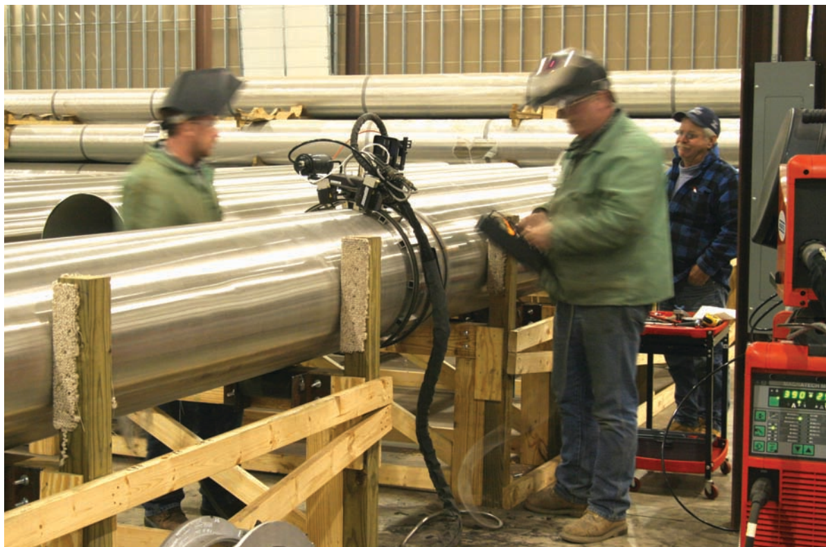
Preparing to weld stainless steel sheathing tubes in the warehouse using a semiautomatic welding system.
