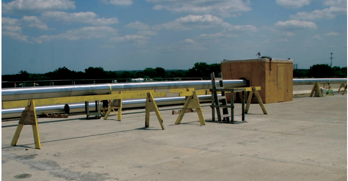
Set-up on bridge deck in Toledo, Ohio, for welding lengths of sheathing together inside site-built work shack.
